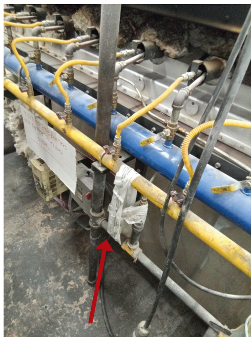
↑ The gas valve handle is secured with cRc tape in a tunnel oven. (cRc tape is tape with the cRc logo used to seal supervised food items and equipment.)
