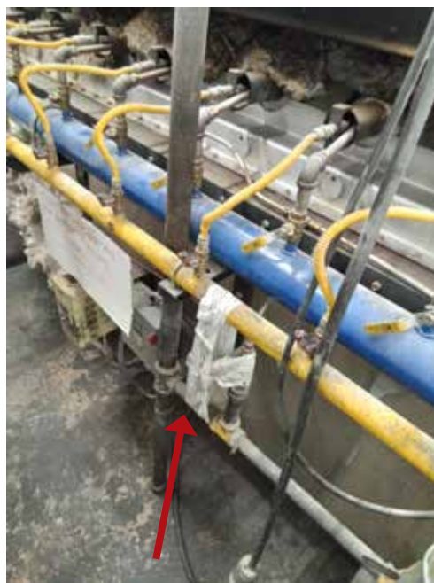
↑ The gas valve handle is secured with cRc tape in a tunnel oven. (cRc tape is tape with the cRc logo used to seal supervised food items and equipment.)
